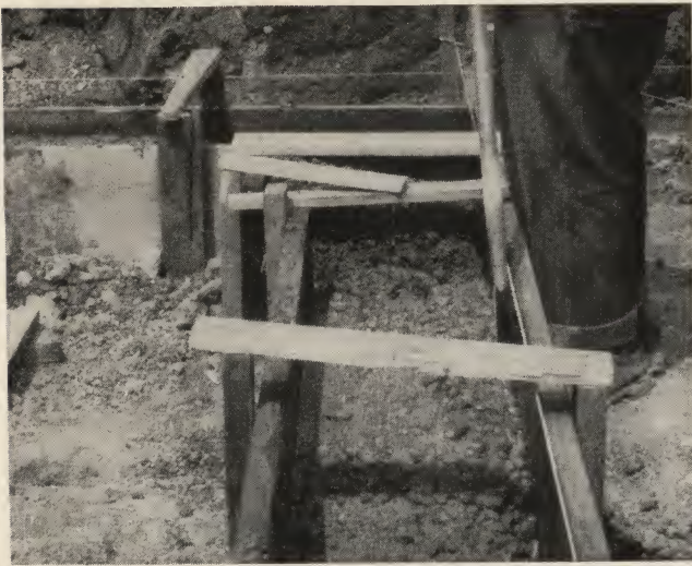
Forms for concrete footings are often made of 2x8 or 2x10 planks as shown here. The stiff concrete mix requires some spading to assure dense, solid concrete.
